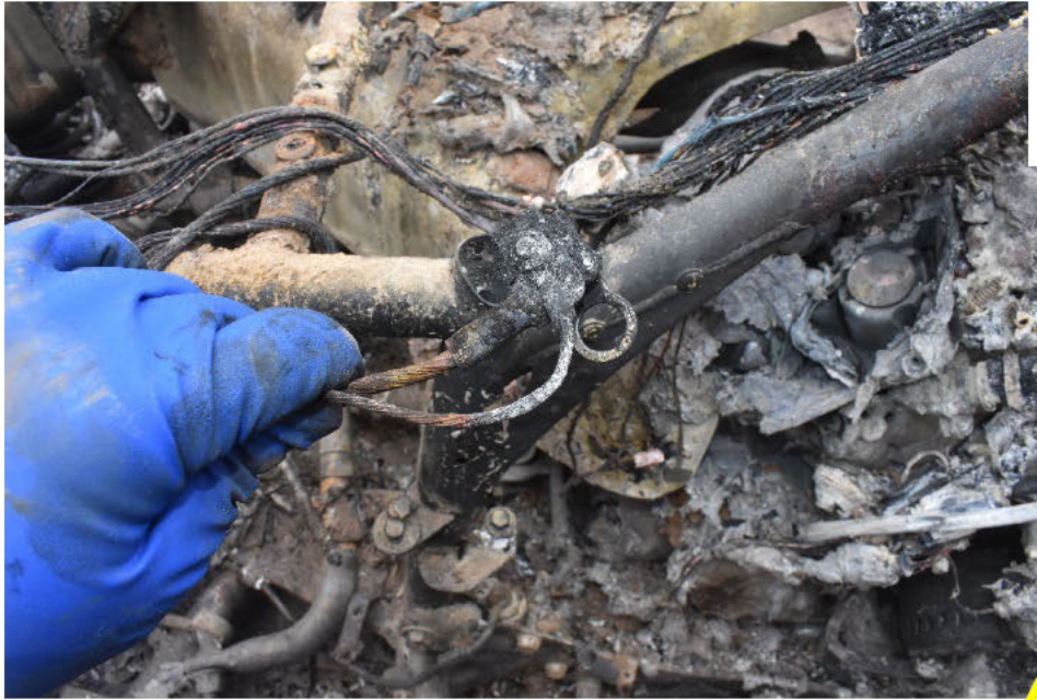
FIGURE 6. FS2025-052 (88), PHOTO OF ARCING ON THE BATTERY CONNECTION.
